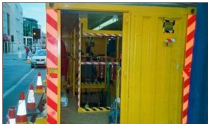
Figure 13 - HV cable jointing container
